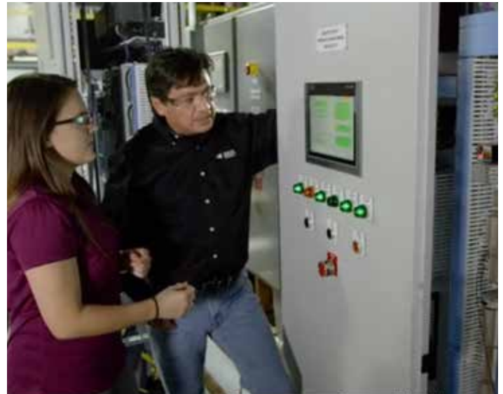
BURNER CONTROL SYSTEM
