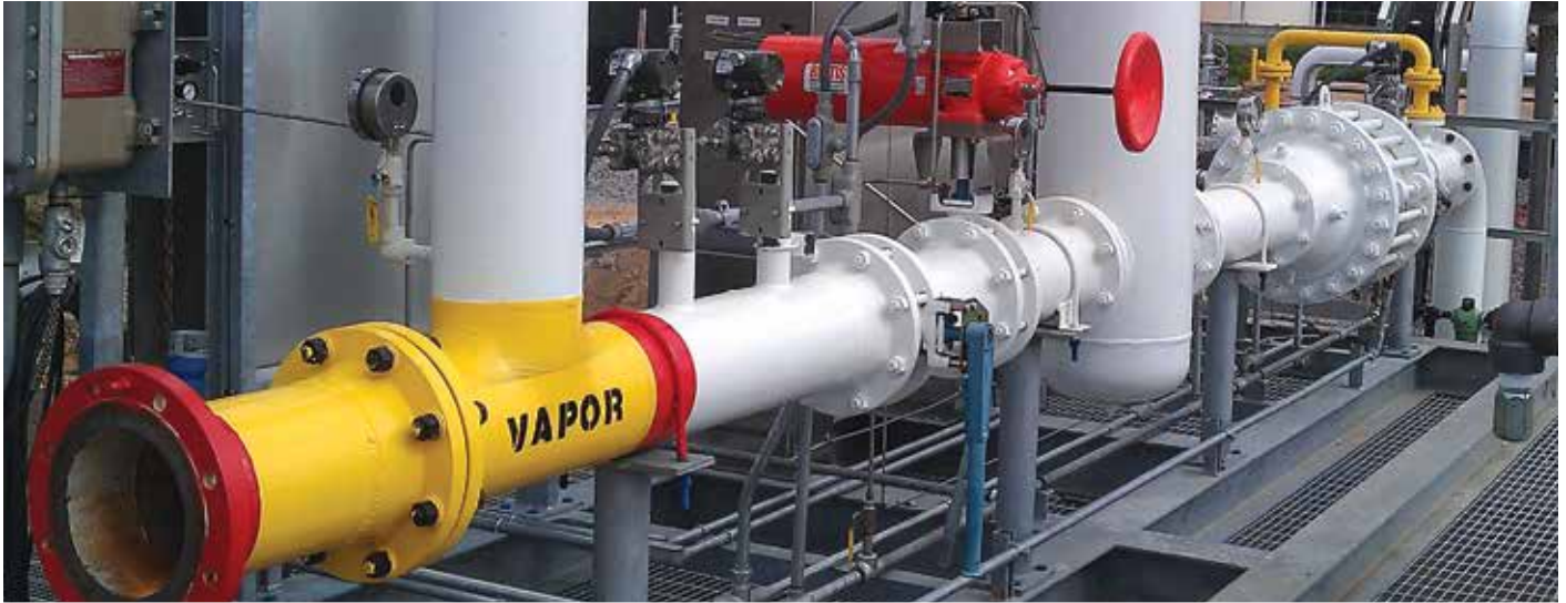
DOCK SAFETY UNIT
