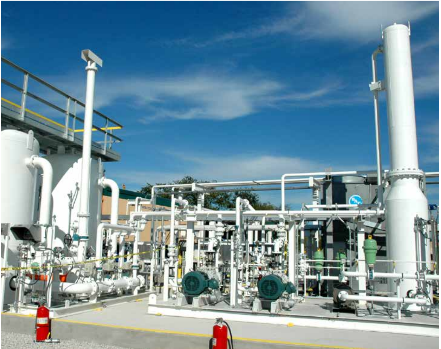
VAPOR RECOVERY SYSTEM
